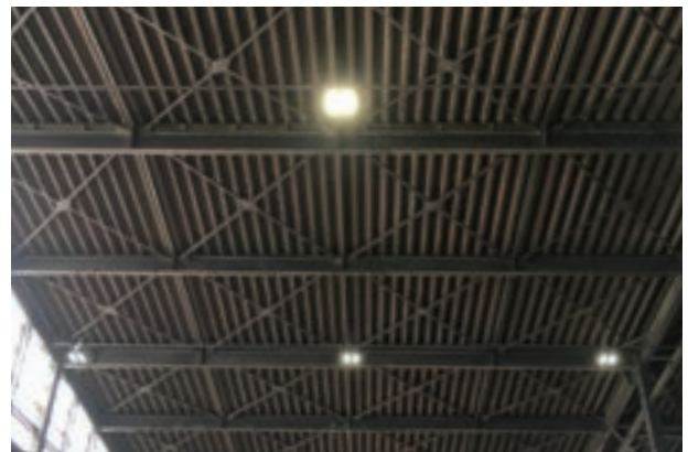
LED light bulbs in Chiba Works
